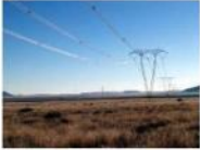
765kV Transmission Pylon @ 1000m
