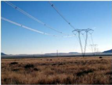
765kV Transmission Pylon @ 500m
