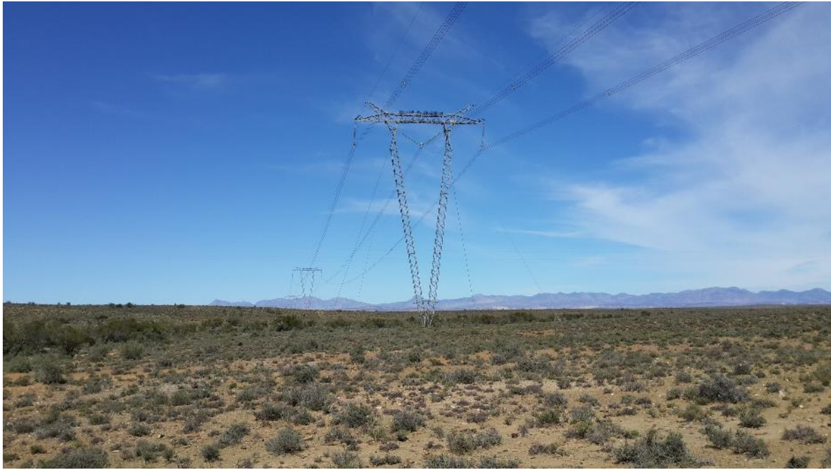
Figure 4: The Droërivier - Proteus 400kV high voltage line
