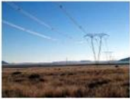
765kV Transmission Pylon @ 1000m
