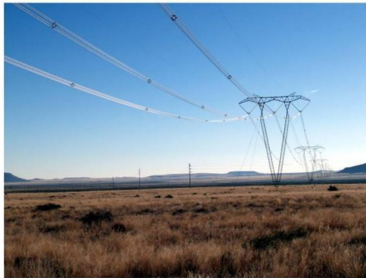
765kV Transmission Pylon @ 250m
