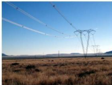
765kV Transmission Pylon @ 500m
