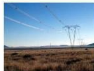
765kV Transmission Pylon @ 1000m
